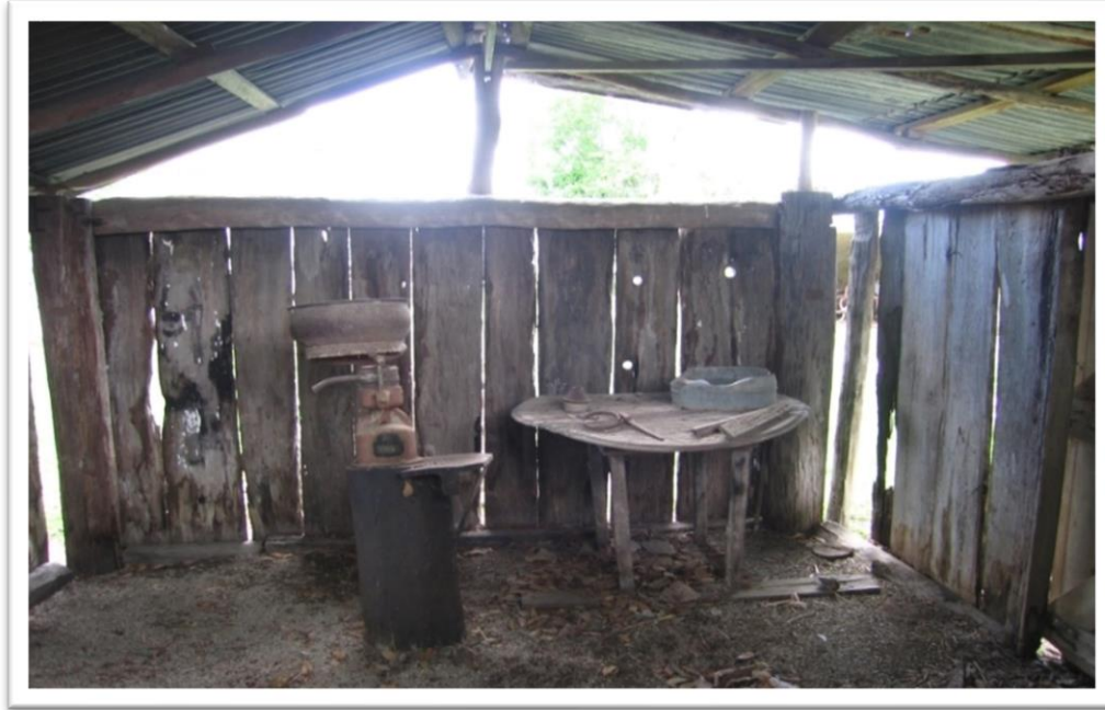
Plate 6.6: Some of the holes in the walls of the Hamilton Station ‘dairy’ are visible in this photograph. The high holes are to look through and the low holes to shoot through. These reoccur around the walls. The boards may once have been part of a larger building, as similar boards with knotholes seem to have been included in what became the slaughterhouse for Hamilton station.
